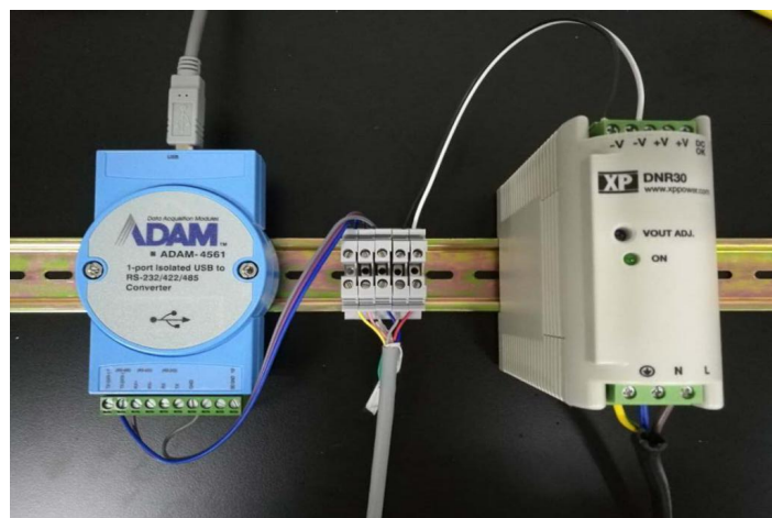
Figure 3.1 Power Supply and 485 converter
